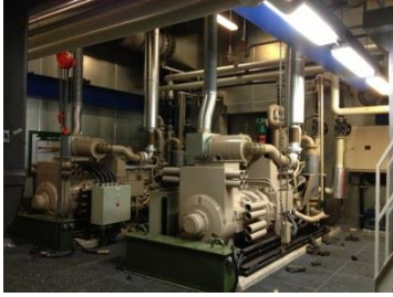
Generators in the bunker
